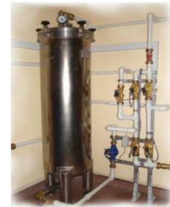
water purification and demineralization plant "KASKAD"
